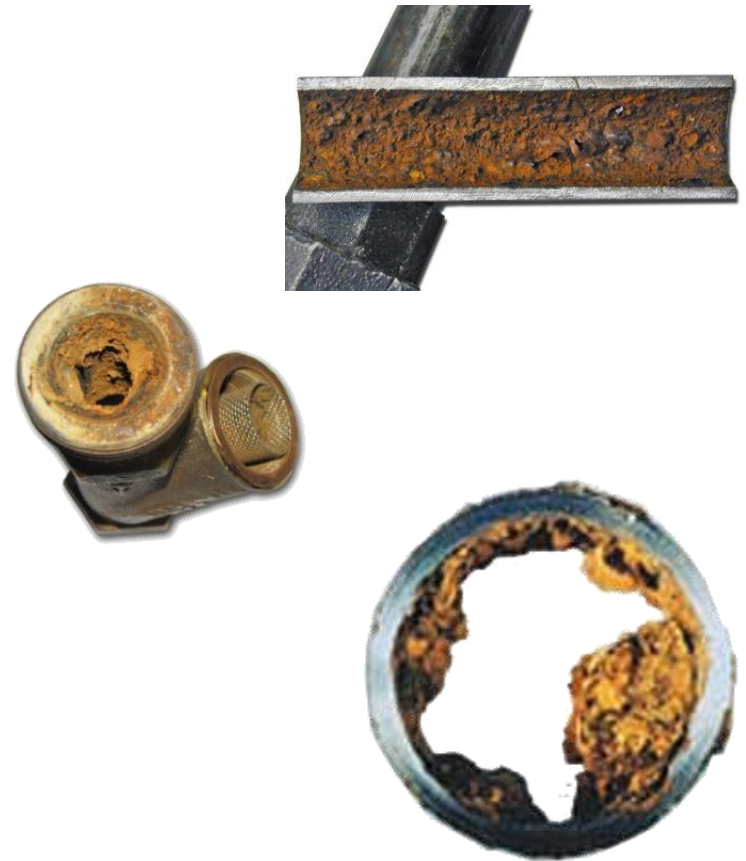
Corroded traditional piping system components
